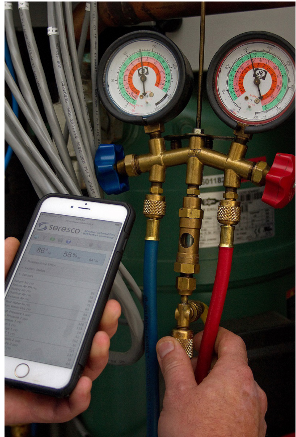
Mobile controls allow remote monitoring of air quality and temperature, and facilitate trouble-shooting.
